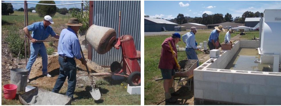
Many hands making light work. Core filling working bee Fuel Facility November 2011.
